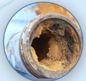
CLOGGING OF PLUMBING PIPES OVER TIME
